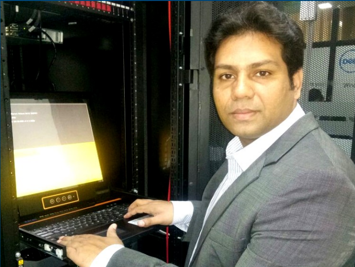
Mr. Danish Qadir Network and System Administrator) is working to configure the servers and Storage Area Network in Data Center.
